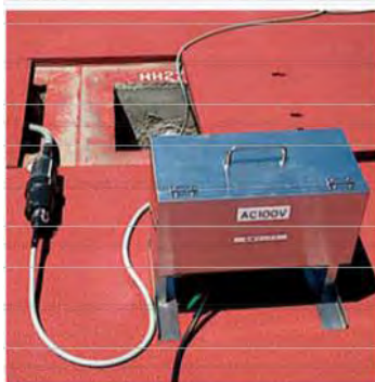
Power cable from sub hand hole is connected to connector box for AC power supply
