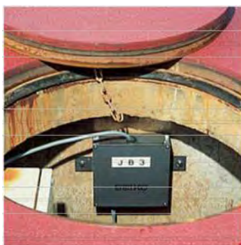
Junction box installed in hand hole
