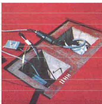
Sub hand hole for signal and power cables
