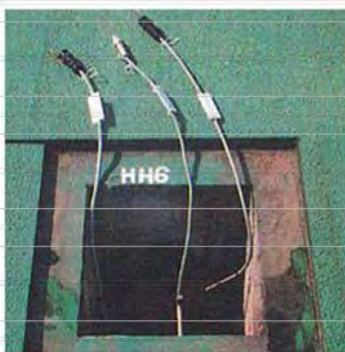
Cable connected to computer terminal (center)
