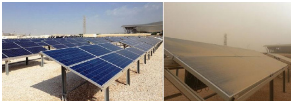
Figure 1. Solar panels before and after sandstorm accumulation
