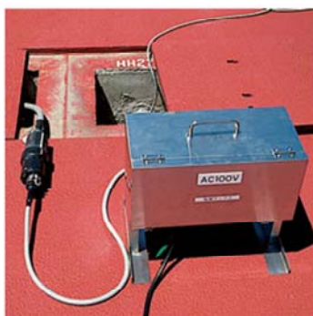
Power cable from sub hand hole is connected to connector box for AC power supply
