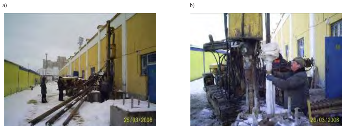
Fig. 9. Well boring (a) driving anchor bars in textile membrane according to author's certificate No 1392203; (b) Borisov
