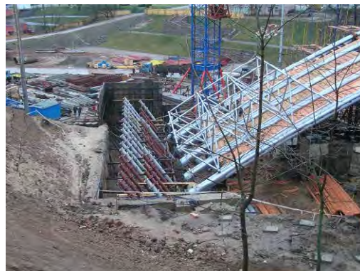
Fig. 5. Pipe arrangement in Fn1 in Vitebsk
