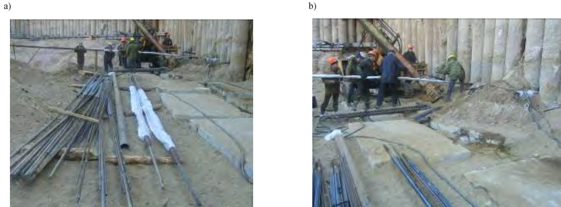
Fig. 4. Assembly of anchor bars according to author's certificate No 1392203 at the bottom of foundation pit (a) and sinking of bars into the hole (b)
