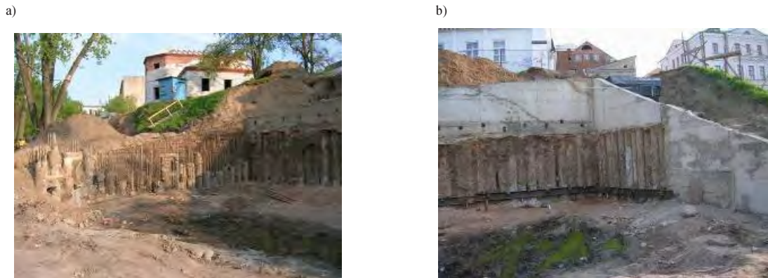
Fig. 6. International street, Minsk: a) excavation near the pile wall on the first tier; b) on the second tier
