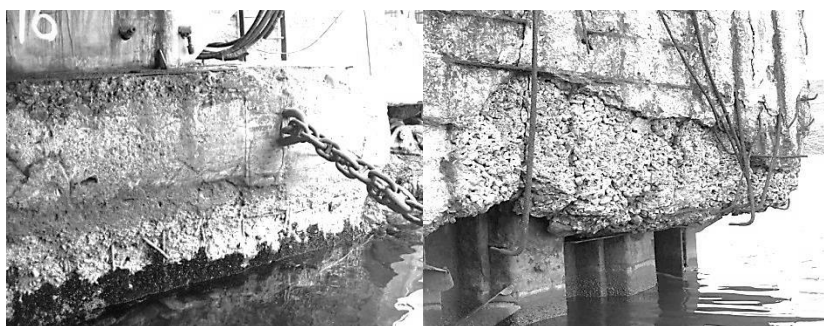
Fig. 2. Quay wall deterioration in a) Kholmok; b) Korsakov port
